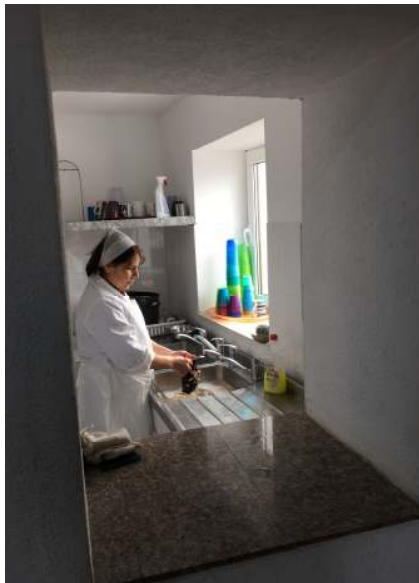
↑ Simona washing up at new sink area, with new granite worktop! ← New flooring laid, and new cupboards built.
